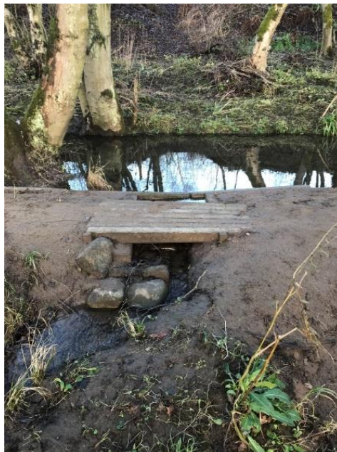
Pond and leaky dam outlet
